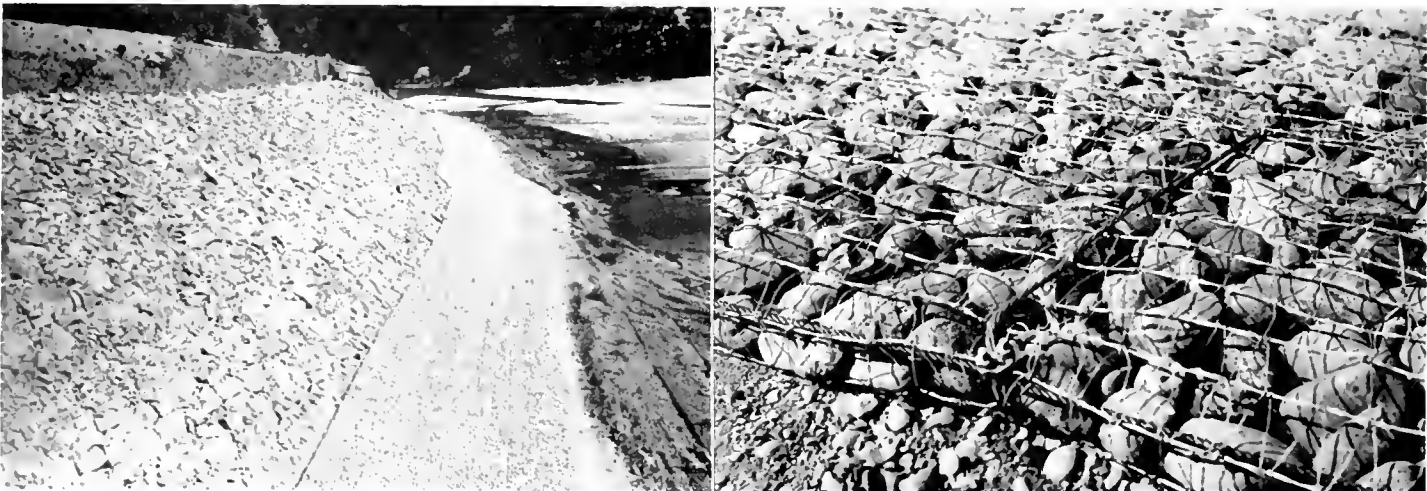
Rock riprap and wire mattress protection of left bank of Eel River below Dyerville. Left: general view, looking downstream Right: detail of mattress and cable tie.
